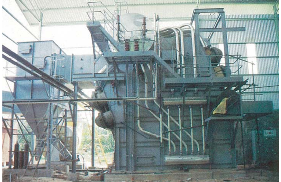
A 35,000 PPH boiler installed in a large timber drying plant in Klang
